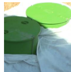
When the tanks are buried to the last 20 – 30 cm from the terrain lay down the geotextile
