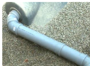
Carefully bury the pumping station with the correct gravel of 4 – 16 mm granulation
