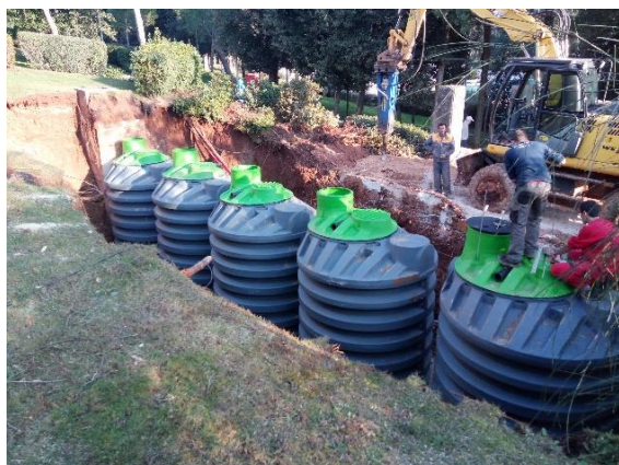
Picture 5: Installed tanks in a row
