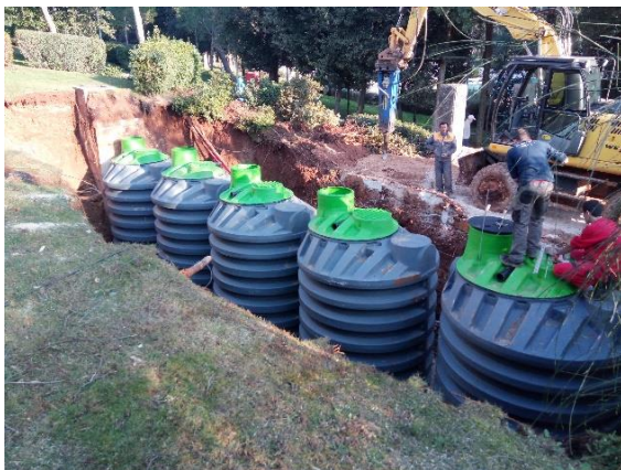
Picture 5: Installed tanks in a row
